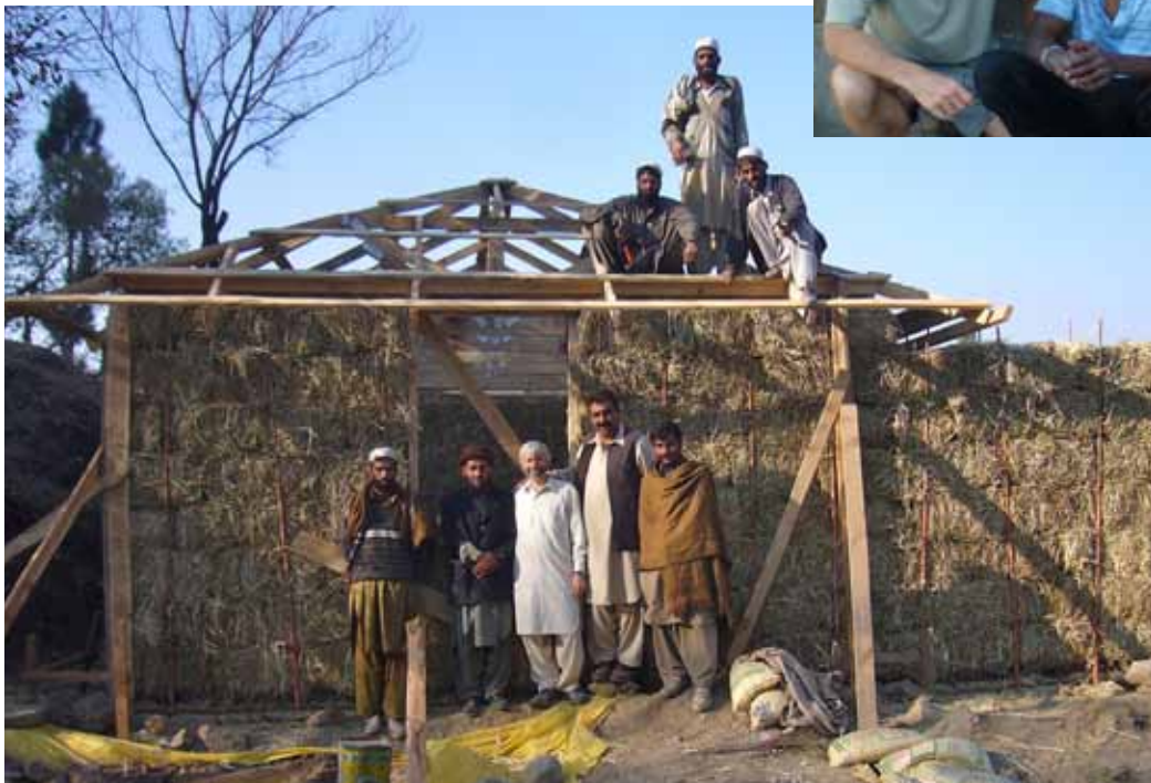
ABOVE: At a straw-bale construction site in Pakistan – Martin Hammer is standing third from the left.
